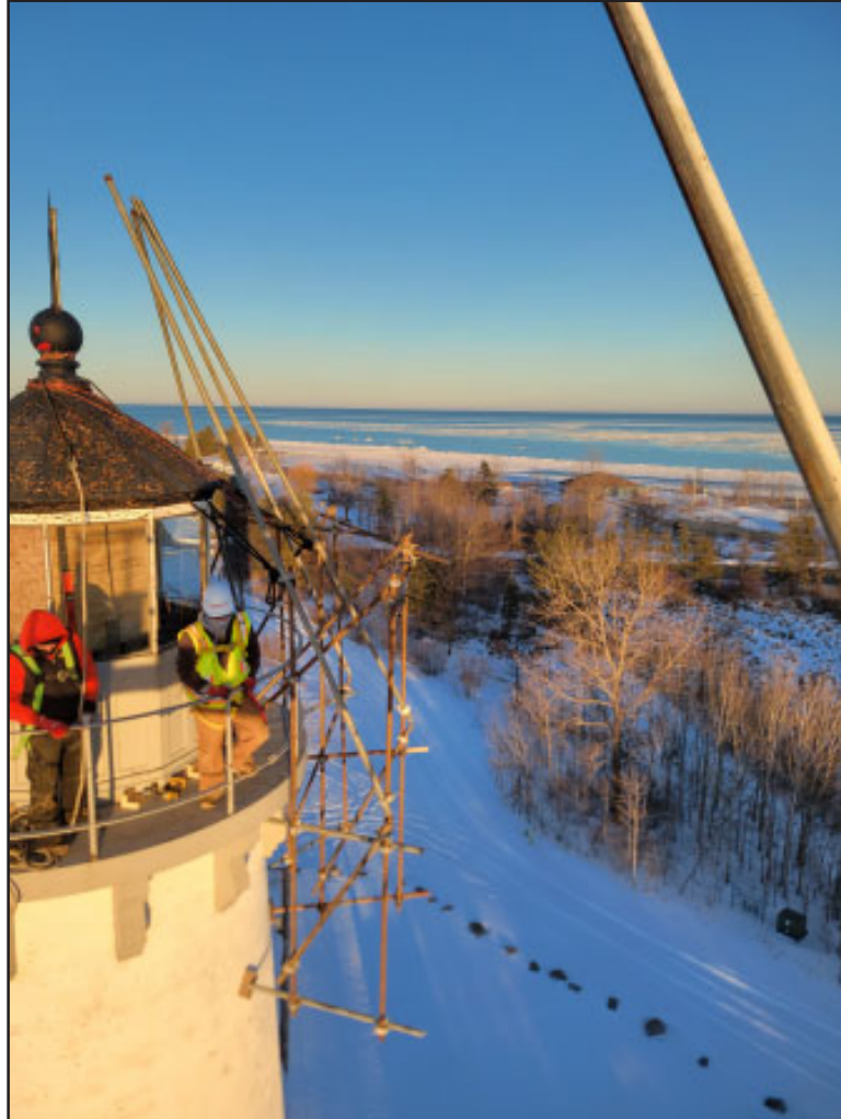
Work began in early 2023, before the snow had melted. Here, workers install scaffolding around the top of the tower in March. Photo courtesy of Mihm Enterprises, Inc.
