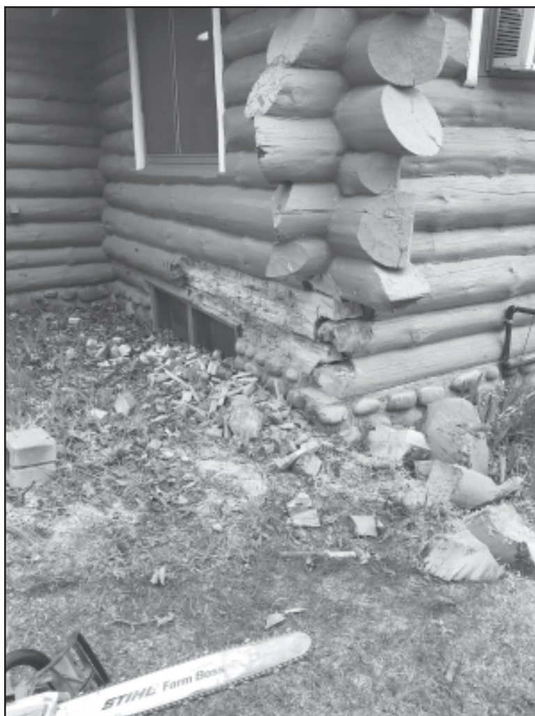
American Log Restoration of Freemont, Mich. completes the replacement of 21 lineal feet of half logs and 28 log ends and one purlin the last week of April. The Craftmakers' Cabin was built in 1936-1937 by the W. P. A. It is owned by the City of Harrisville and leased to the coop of artists and crafters known as The Craftmakers' Cabin. Courtesy photo.
