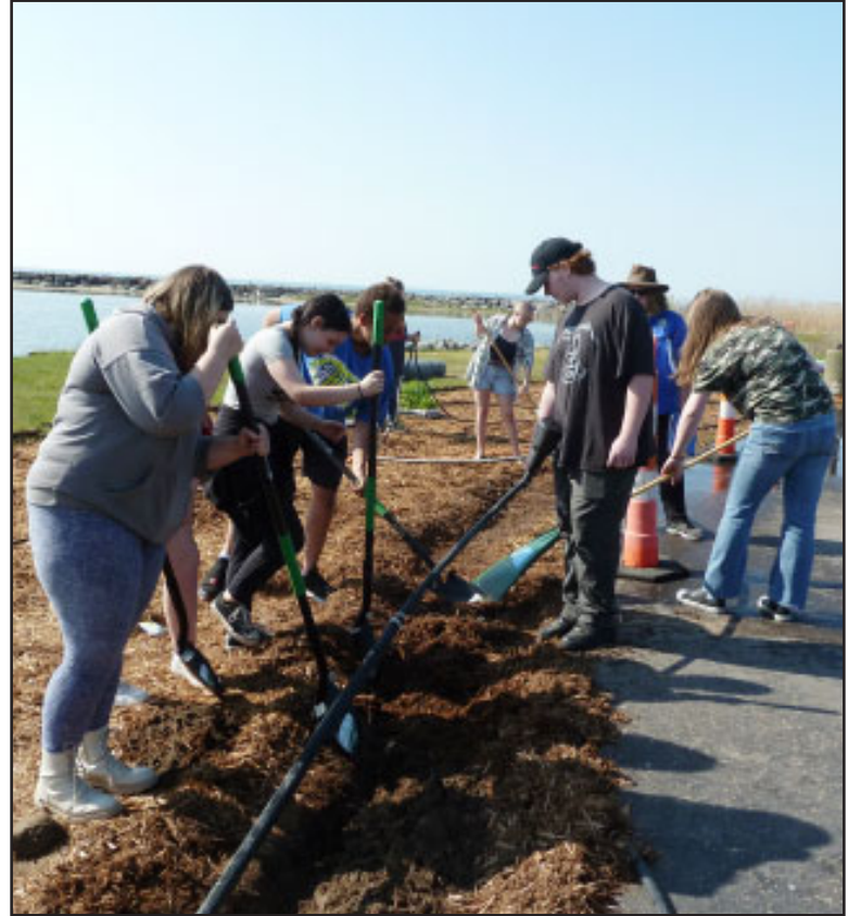
Alcona High School Environmental Science teacher, Kathrin Luce (front left) works alongside her students digging to install an irrigation hose at the rain garden at the Harrisville Harbor of Refuge. The garden, designed by students, was planted to catch and filter pollutants before they enter Lake Huron. The project was funded by a combination of entities. (Left to right): Kathrin Luce, Piper Fletchinger, Isabella Bravata, Danica Manning, Jayson Lincoln, Aiden Reno, and Sarah Morris from NEMIGLISI. Photo by Mary Weber.
