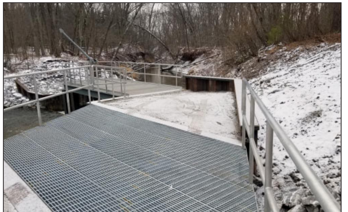
This permanent $1.67 million sea lamprey trap was completed on January 24. The project represents a long-standing partnership between U.S. Army Corps of Engineers, Detroit District and Great Lakes Fishery Commission to control invasive sea lampreys and protect the $7 billion Great Lakes fishery from the parasitic fish species. U.S. Army Corps of Engineers Photo by Adam Virga.
