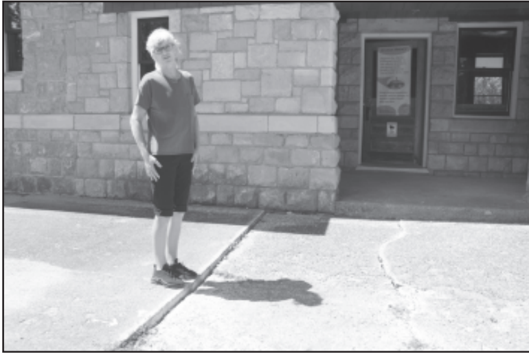
Becky Schroeder is hoping someone who knows concrete could come up with a solution for the cement that is crumbling around the exterior of the depot. Photo by Mary Weber.
