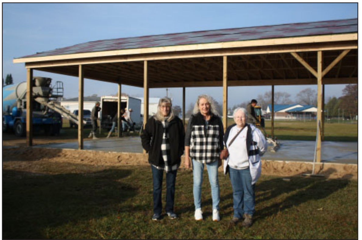
Marsha Mahalak (left), Linda Somers (center) and Sheila Philips are all smiles as they watch the construction of the "One Dime at a Time Pavilion" next to the Flight of Imagination Playground in Lincoln. Photo by Mary Weber.
