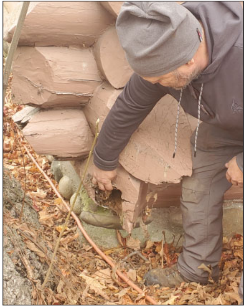
Angel shows where logs are in decay in the 85-year-old log building which has housed The Craftmakers' Cabin cooperative for the last 40 years. Photo by Mary Weber.
