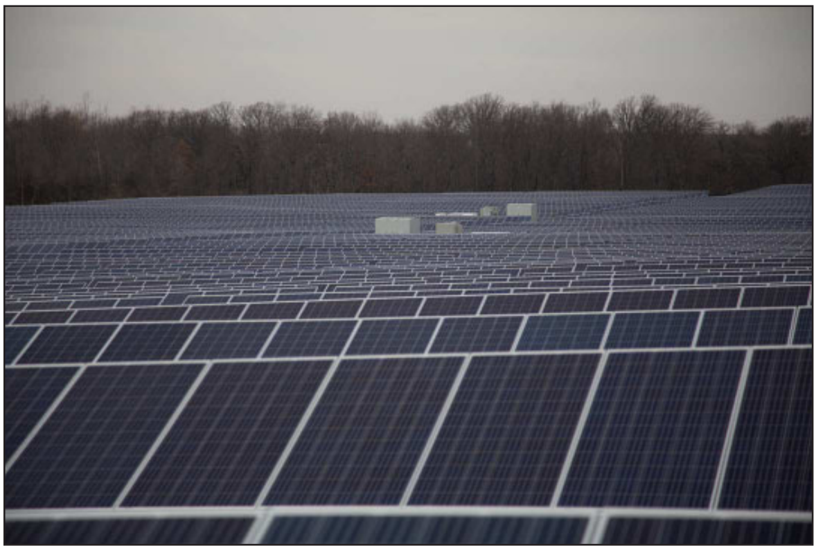
This DTE solar panel farm is located in Lapeer, Mich.
