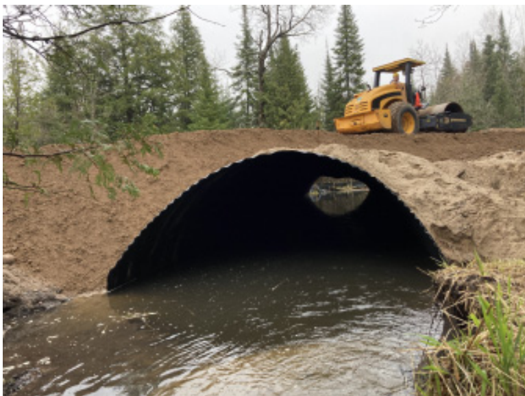
The new culvert where Kimberlin Road crosses Kurtz Creek is more than 14 feet wide, allowing for natural stream flows and fish passage.
