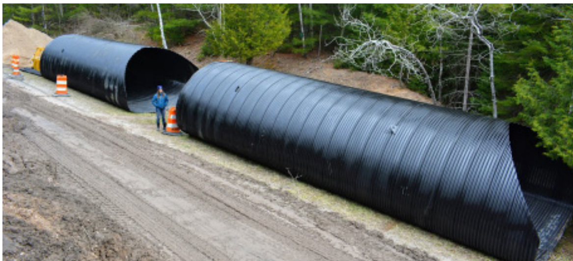
The new culvert was delivered to the site in two pieces and staged for installation. Amy Nowakowski, Coastal Project Manager for Huron Pines, the nonprofit organization heading the project.
