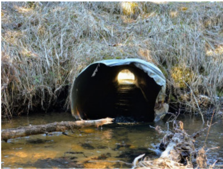
The former culvert at the crossing of Kurtz Creek at Kimberlin Road. Photos courtesy of Huron Pines.
