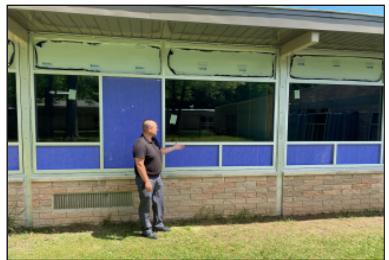
Superintendent Dan O'Connor outside Alcona High School where new windows will be installed in place of the purple insulation that is protecting classrooms. Courtesy Photo.
