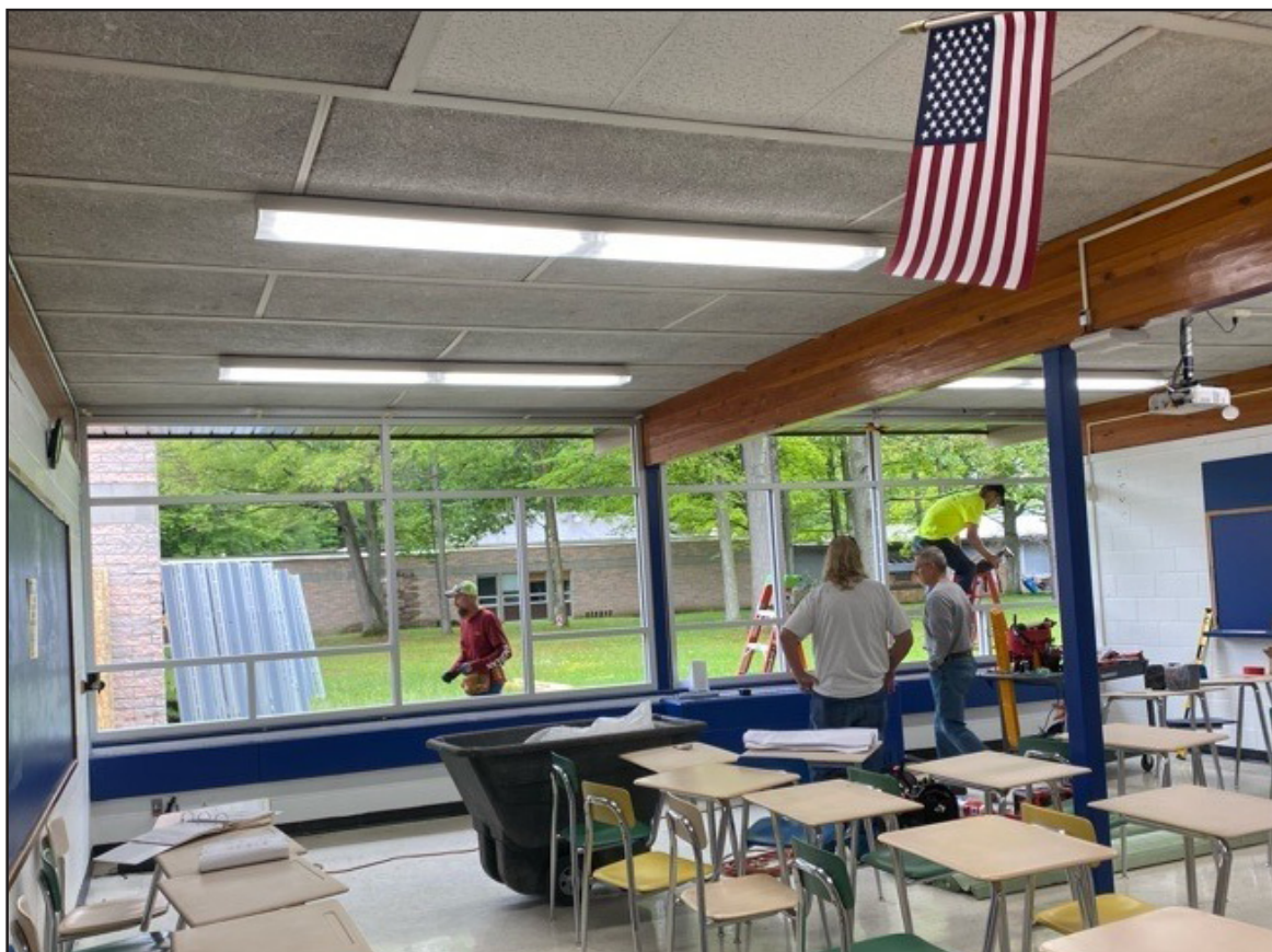
Contractors remove old windows in the high school and middle school this summer in preparation for new, more energy efficient and safety conscious windows. Courtesy photo.
