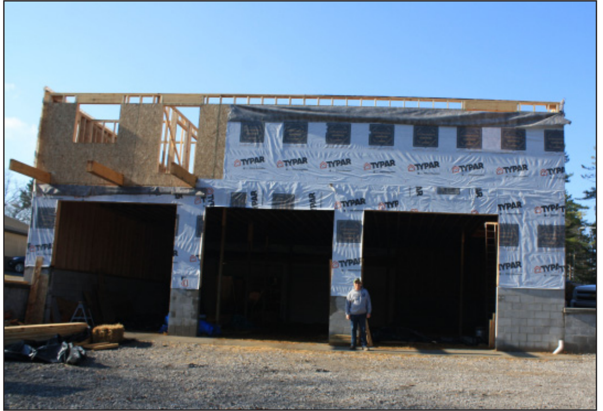
Barton City Fire Chief Rod Cordes stands in front of the three large bay door openings of the fire hall expansion.
