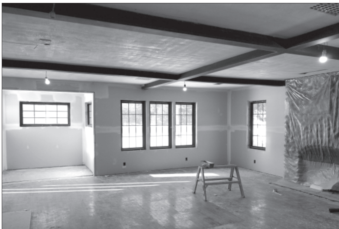
Remodeling work resumes on Alcona Brew Haus located north of Harrisville on US-23. Drywall was completed on January 9 and the interior, including the dining room (above), is ready for paint. For an update see page 4. Courtesy photo.
