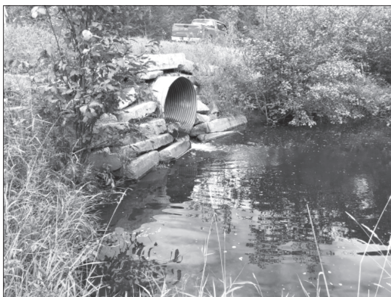
The culvert for Curtis Creek (Wilbur Creek) on Brodie Road is being replaced this fall. Courtesy photo.
