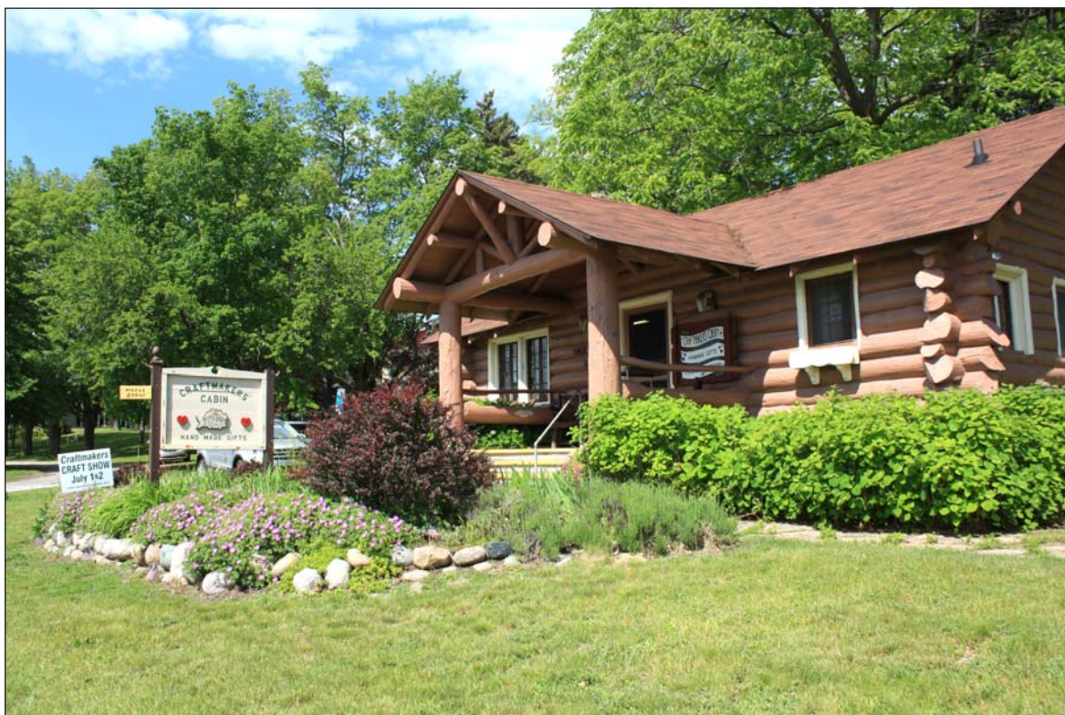
A familiar site in Harrisville, the Craftmakers' Cabin is located on the corner of US-23 and M-72. This 80-year-old log cabin is in need of a new roof and the windows need to be re-glazed. Photo by Mary Weber.
