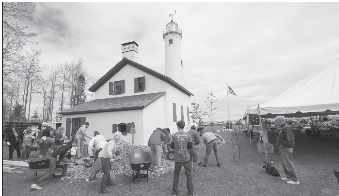
Workers in progress on a repair project at the Sturgeon Point Lighthouse in Alcona County. The project was aided by funding from a Recreation Passport grant.
