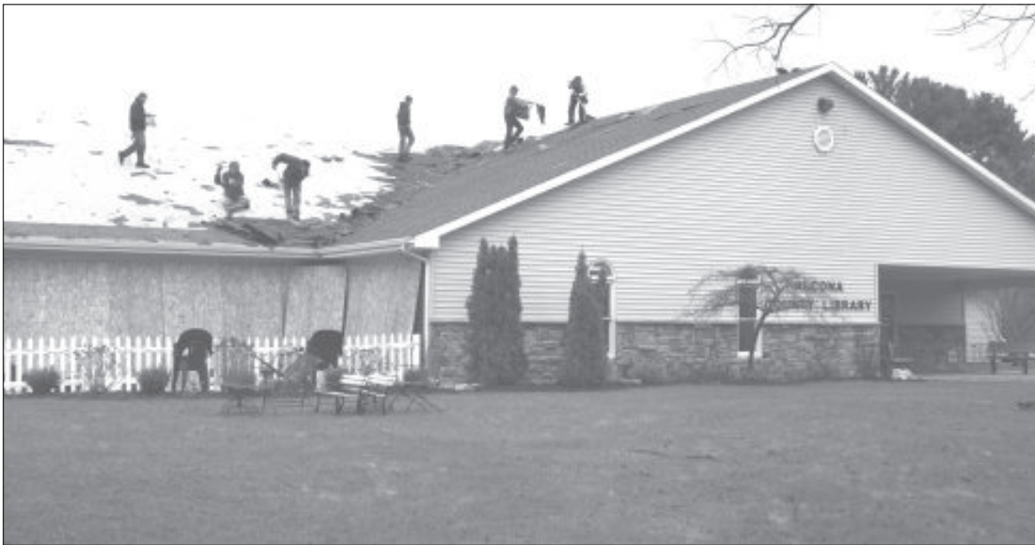
Work on the roof of the Harrisville branch of the Alcona County Library is underway this week. Photo by Mary Weber.
