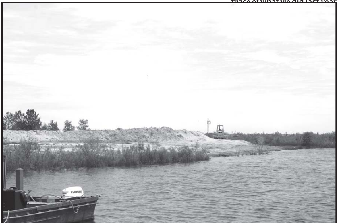
Residue from the dredging project is deposited on state land located north of the harbor until it dries out, then it will be removed and the area will be restored.
