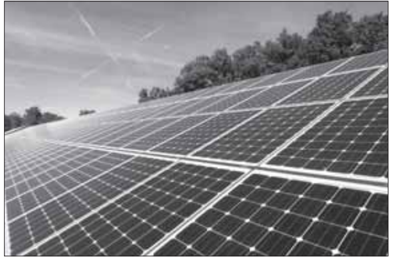
DTE Energy's 1.1-megawatt solar array at Domino's Farms near Ann Arbor, Michigan. Photo courtesy of Mark Houston.
