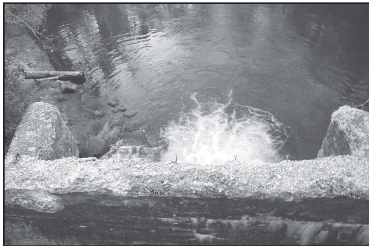
Buhl Dam is slated for removal by the U.S. Forest Service in 2016. Photo by Mary Weber.
