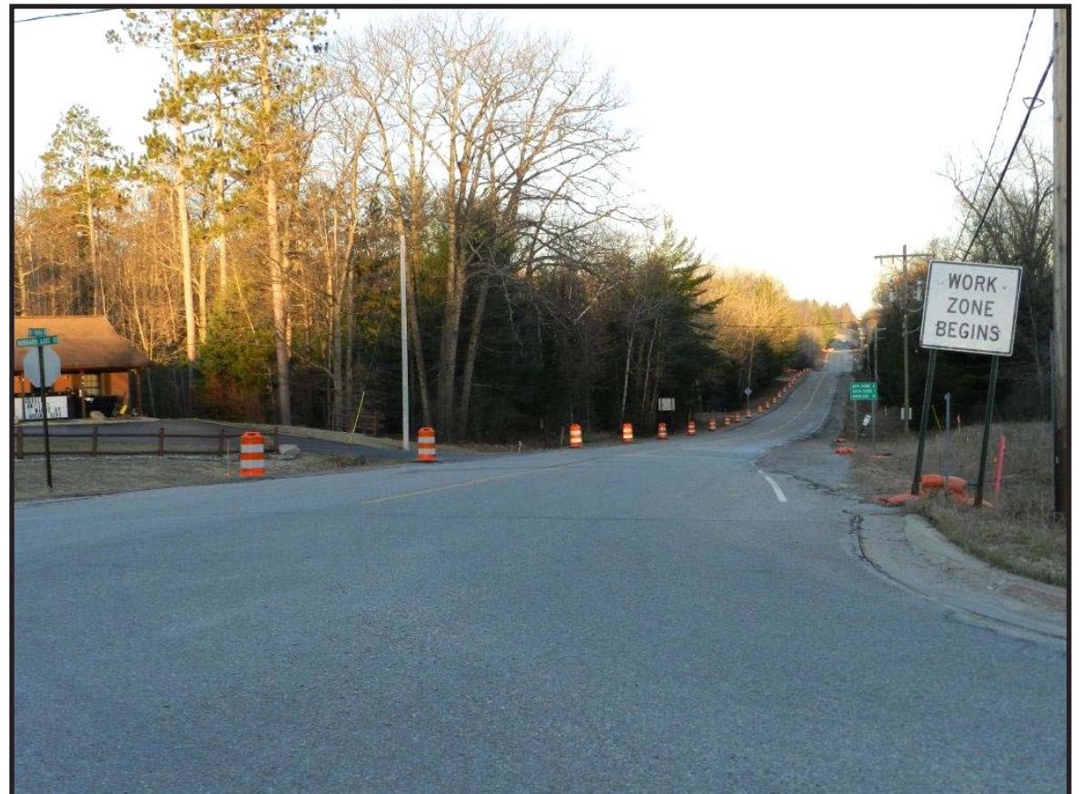
The early morning light illuminates a row of construction barrels standing like sentinels along Mt. Maria Road waiting to be called into duty as road crews are scheduled to begin work there on or about May 1. Courtesy photo.
