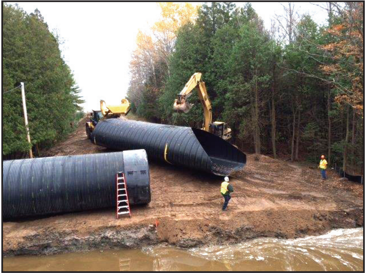
This 96 foot by 14.5 foot by 9 foot culvert was installed on Quick Road crossing Haynes Creek near the end of October by crewmembers of the Alcona County Road Commission. Courtesy photo.
