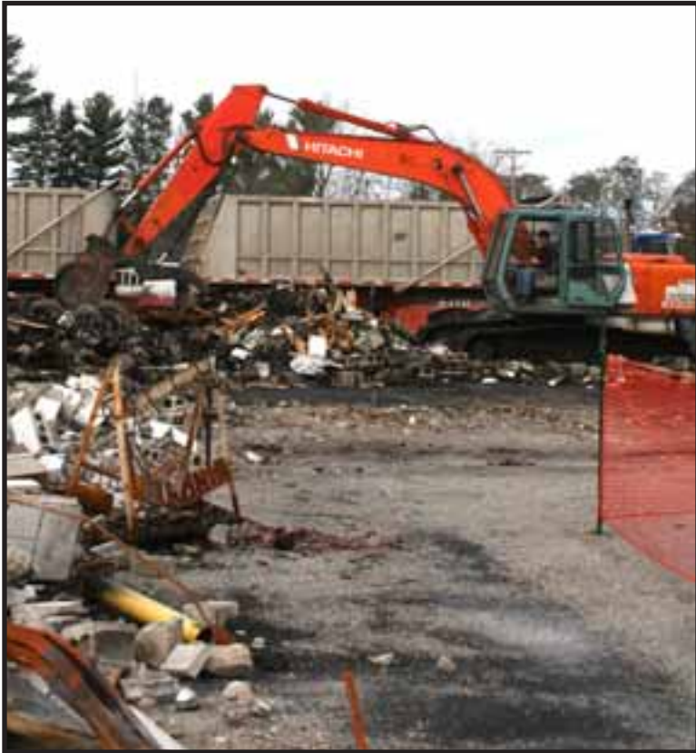
Clean up has begun at the Alcona County Road Commission building one month after it was destroyed by fire. Clean up began October 28; trucks and other large equipment were removed on Monday. Photo by Cheryl Peterson.
