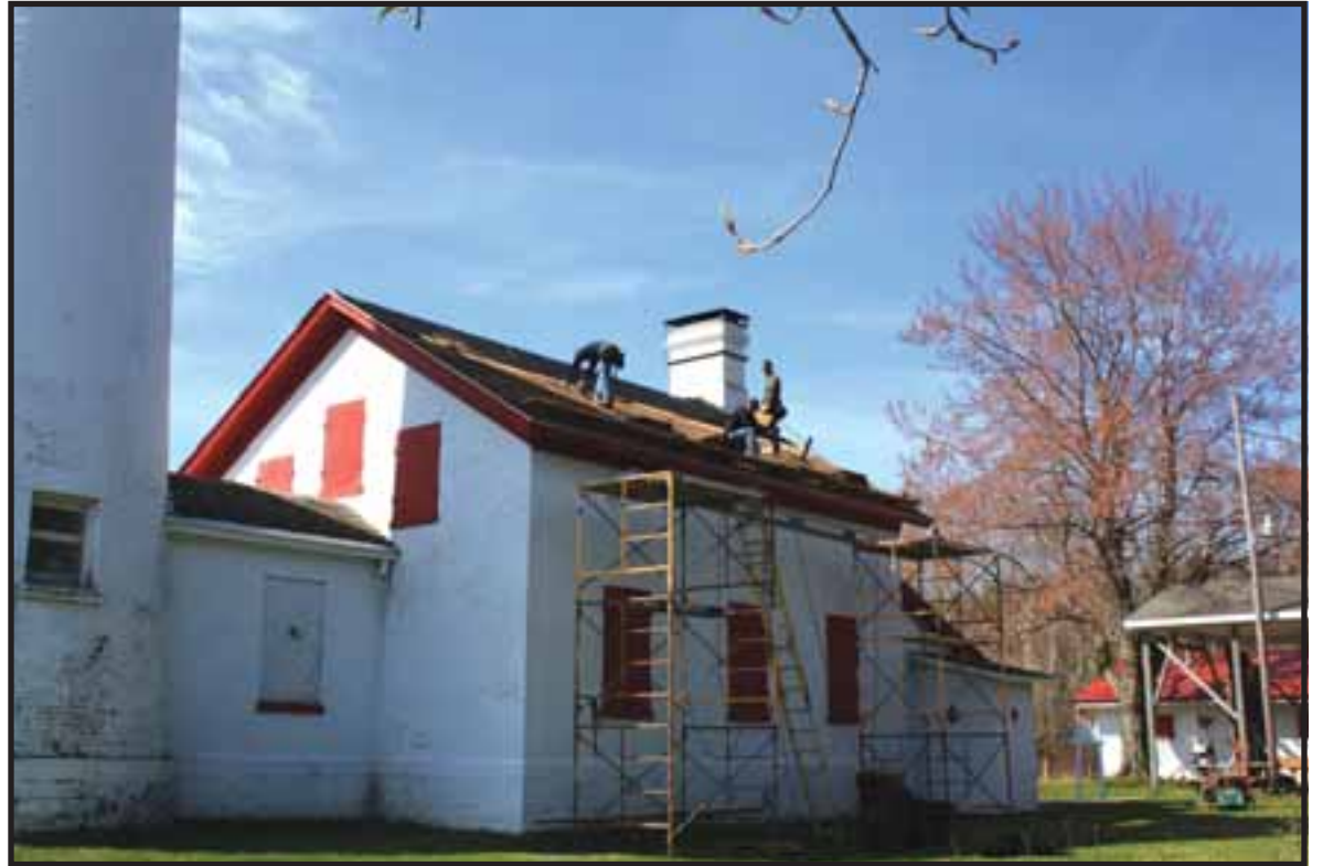
Workers replace the roof of the lighthouse. The old roof was put on in 1979, and is possible from a grant from the Michigan Department of Natural Resources. Photo by Mary Weber.
