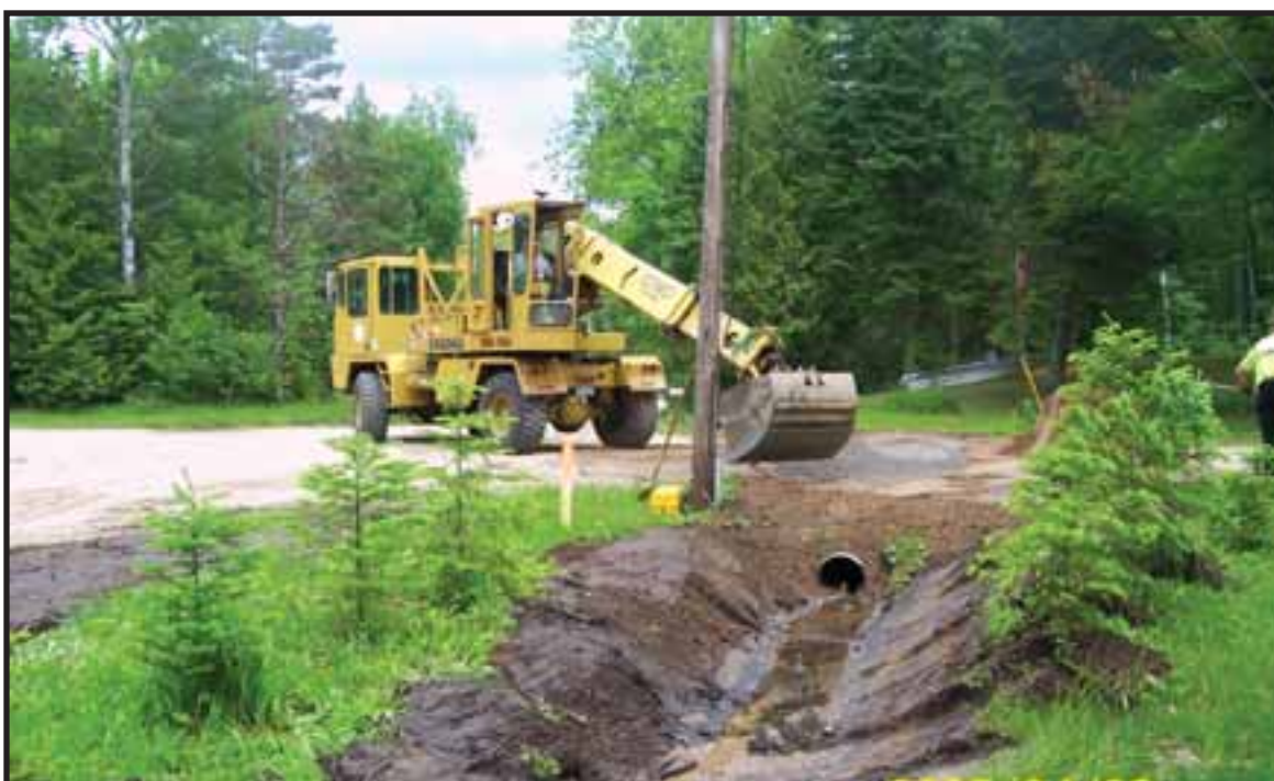
Alcona County Road Commission crews clean out a ditch and replace a culvert to ensure proper roadside drainage. Courtesy photo.
