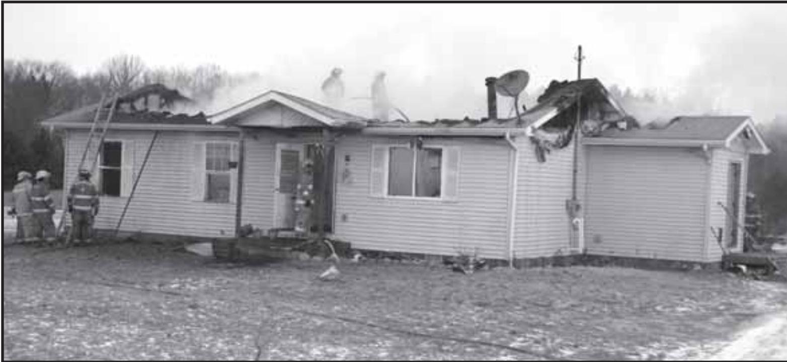
Fire fighters battle an early morning blaze in Lincoln Tuesday. They were called out at 6:35 a.m. to a home near Twin Lakes Cemetery on Trask Lake Road. Those first on the scene found flames through the roof of the dwelling. According to Roger MacNeill, incident command officer and DNR Fire Officer, the family was home when the fire started, but was able to leave without incident or injury. Fire departments from Lincoln, Barton City and Mikado responded to the call as did fire fighters from Harrisville. Photo by Cheryl Peterson.
