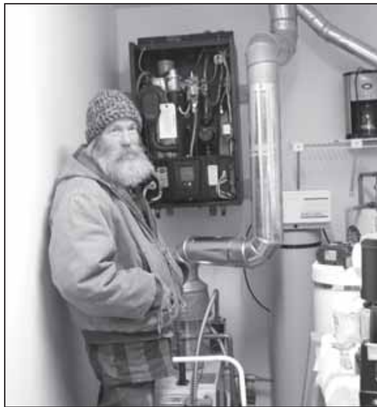
Tom Pyle, of Gauthier Heating and Cooling, mounts a new heating unit in Carol Park's home. Pyle said they regularly test CO levels on furnaces. Photo by Mary Weber.
