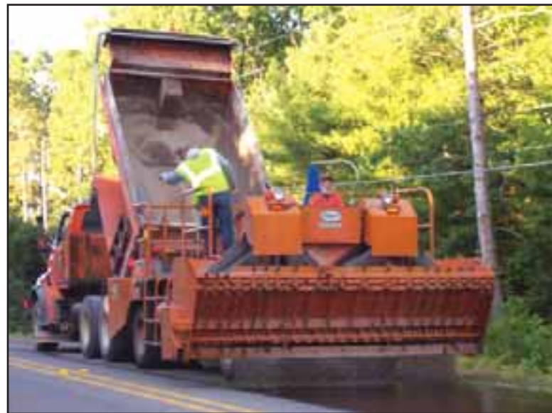
Alcona County Road Commission employees Linton Fowler Jr. (left) and Drew Milwrick work in sync with truck drivers to unload crushed stone into a spreader machine to cover fresh tar. All part of the sealcoat process strategy to extend the life expectancy of a road surface. Courtesy photo.
