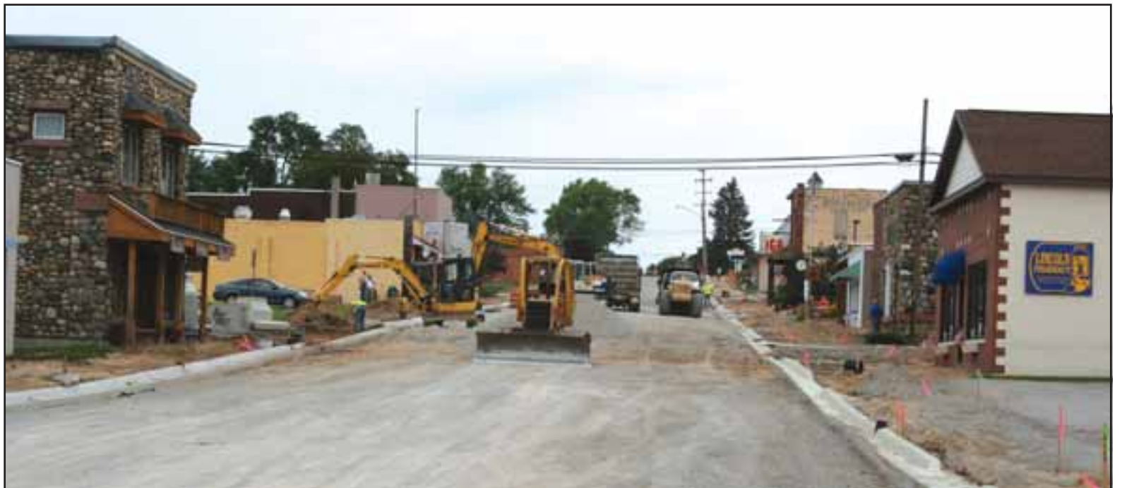
Crews have been working on phase one of the streetscape project on Second Street in Lincoln since early July and will be pouring sidewalks this week. Photo by Cheryl Peterson.
