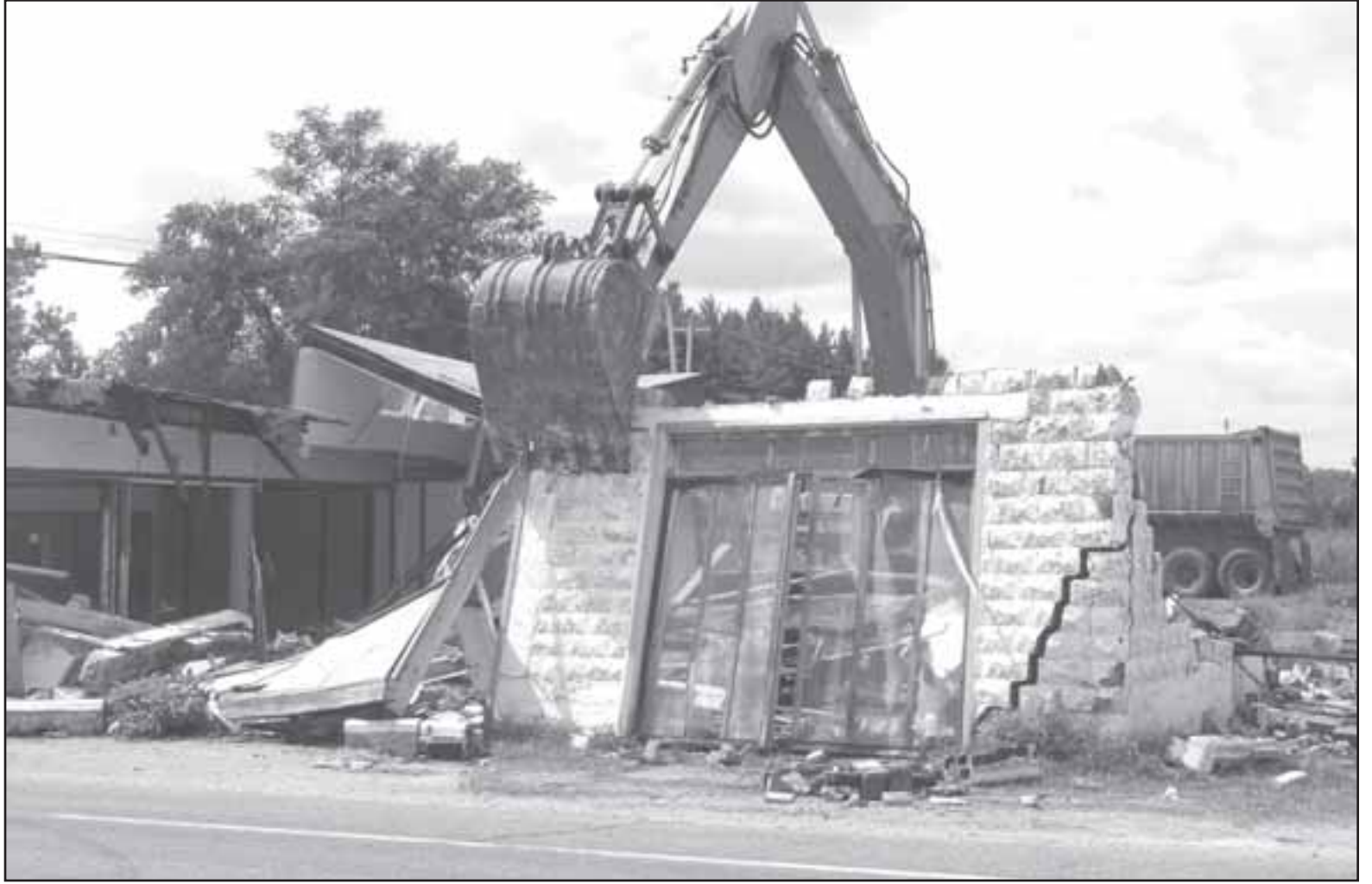
Demolition of the building on the corner of F-30 and F-41 was underway around 1 p.m. Tuesday. Photo by John Boufford.
