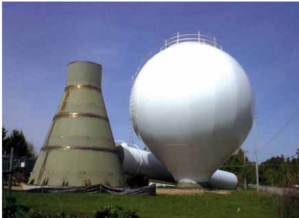
Construction of the City of Harrisville's new water tower is moving along. Photo by Art Kniep.
