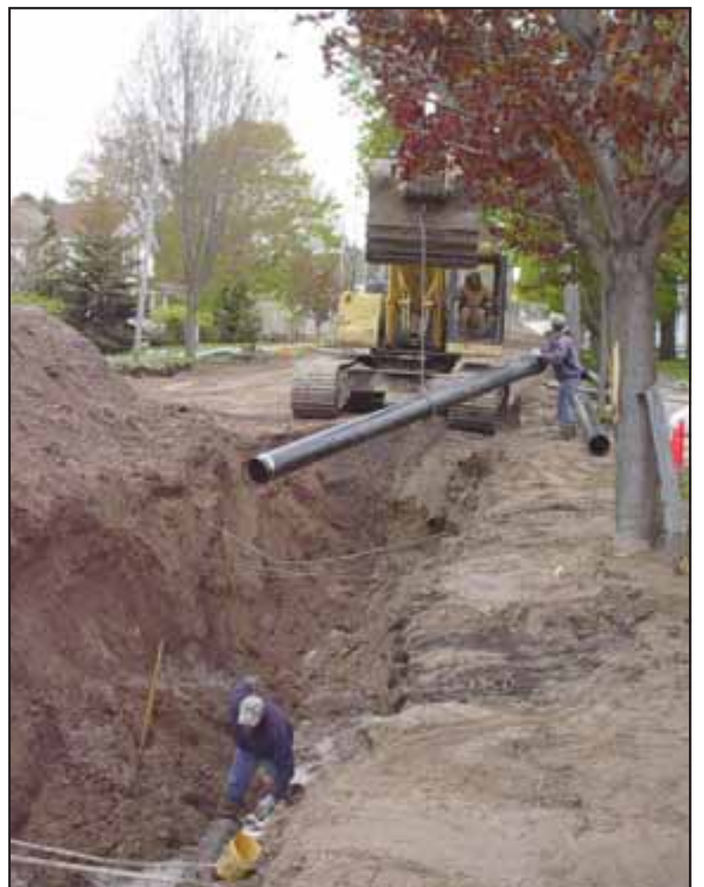
Workers put in the main water line on Main Street at the third block in Harrisville Tuesday morning. Photo by Art Kniep.
