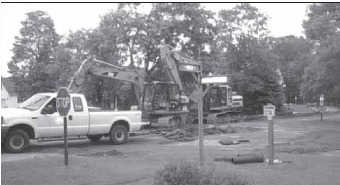
Harrisville's ongoing water main replacement project has moved from Main and Lake streets to side streets. Pavement is being removed on the corner of Dock and Lake streets. Photo by Art Kniep.
